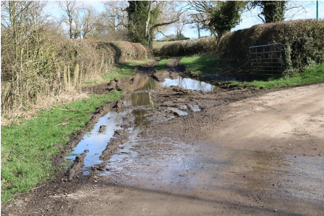
Unsurfaced section of High House Lane, looking north east
