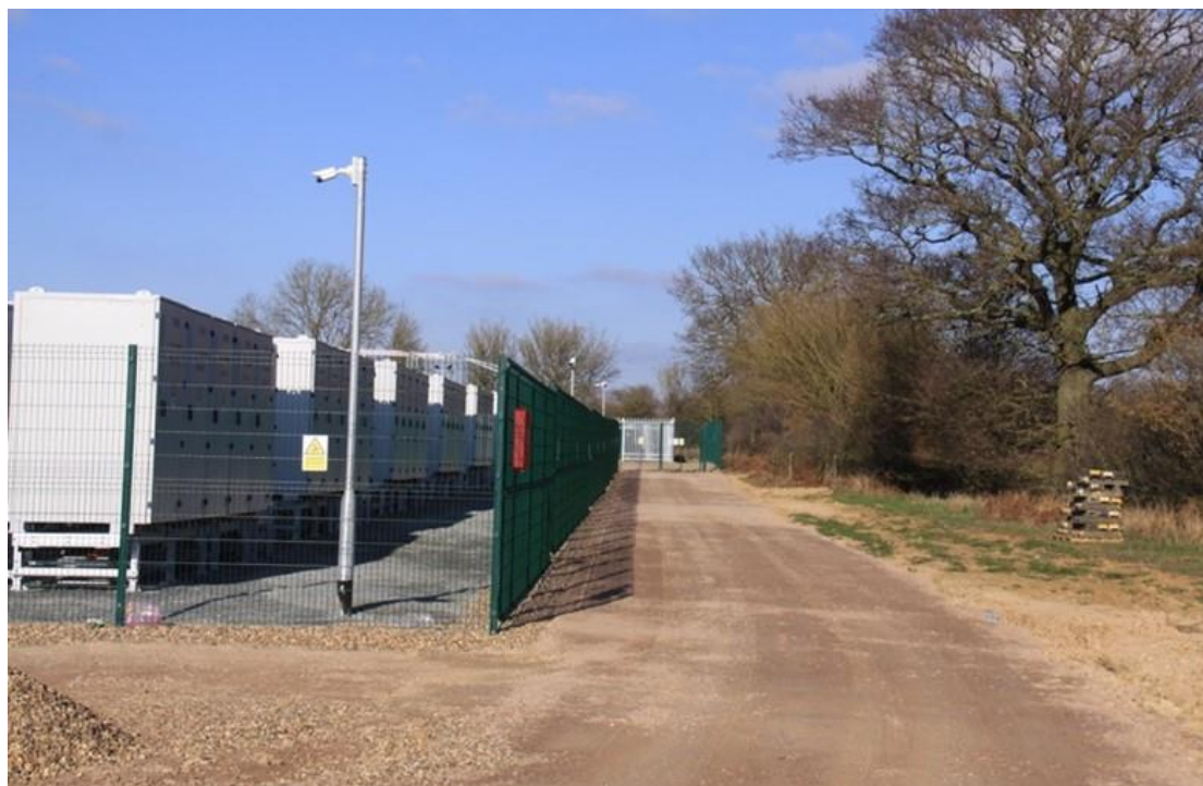
LLPS 17 fencing at BESS site
